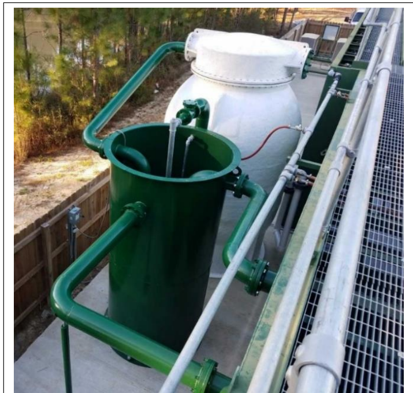
Figure 8. An HPPG can be configured with a recirculating aeration tank to become an effective bioclarifier, nitrifying and reducing soluble BOD while capturing solids.
